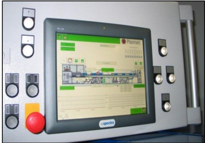
Figure 4. PLC controls with Siemens HMI
